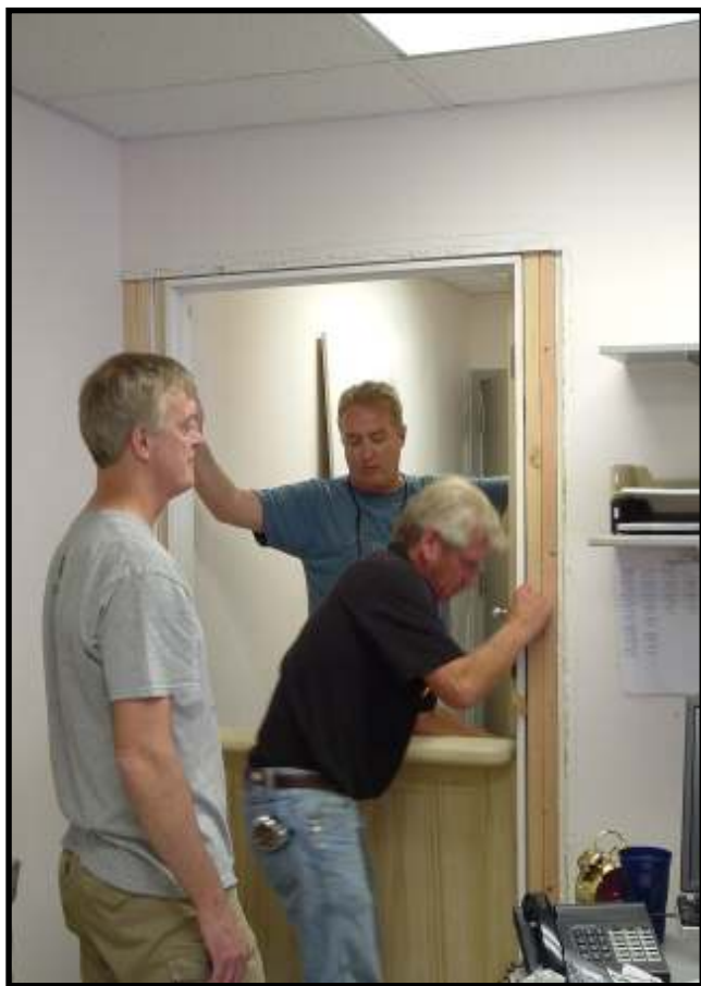
InterFaith's medicine dispensary gets a facelift with the installation of a new door to be used for dispensing. InterFaith is grateful to Mike Torrey, Garrett Hanas, and Bill Torrey for donating their time to install the door.
